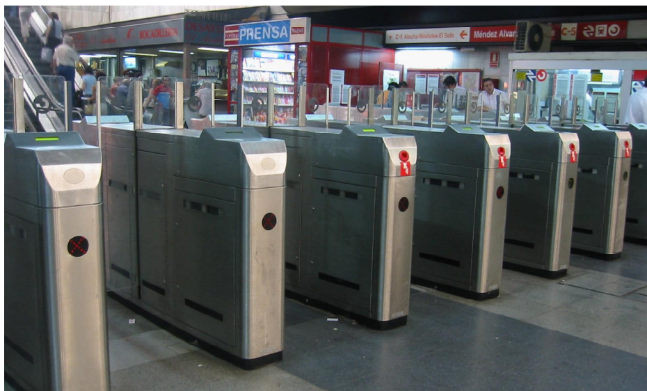
Flap control gates
