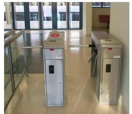
Turnstiles control gates
